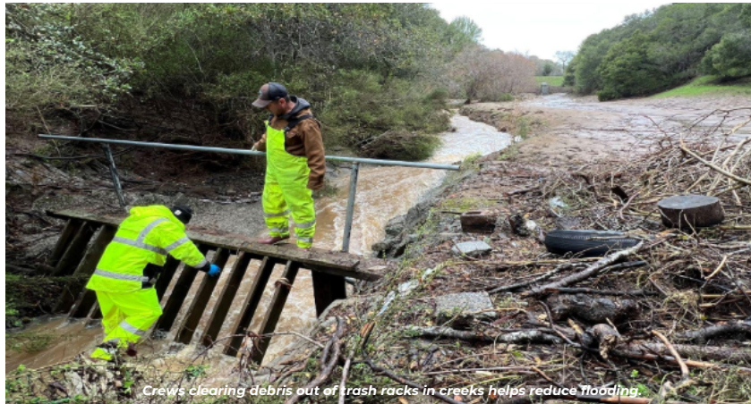
Crews clearing debris out of trash racks in creeks helps reduce flooding.
